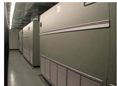
Three 30 Ton AC Units, More Than Double the Need
