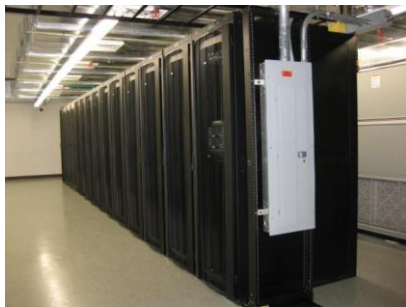
One of Three Rows of Individually Secured Racks
