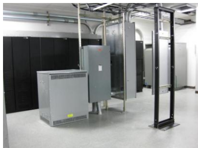
Transformers & UPS's for Each Rack and Row
